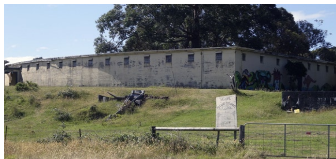
The vandalised and deteriorating rear of the prison, 2014, then the McLeod Eco Farm and shut to the public. Photo by editor.
