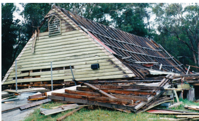
The same building five days later, on the 29th April 1995. Photo by Jan Walker.
